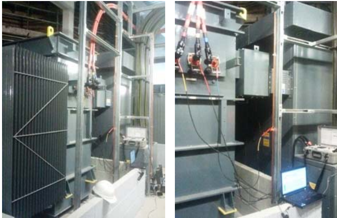
Figure – 6: Tests on the Rectifier transformer using the Three Phase TTR tester for ratio and phase shift.
